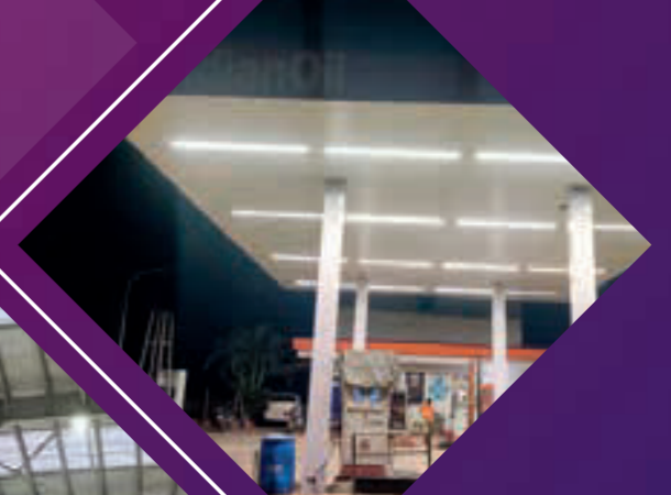
Petrol station lighting, Erode, TN
